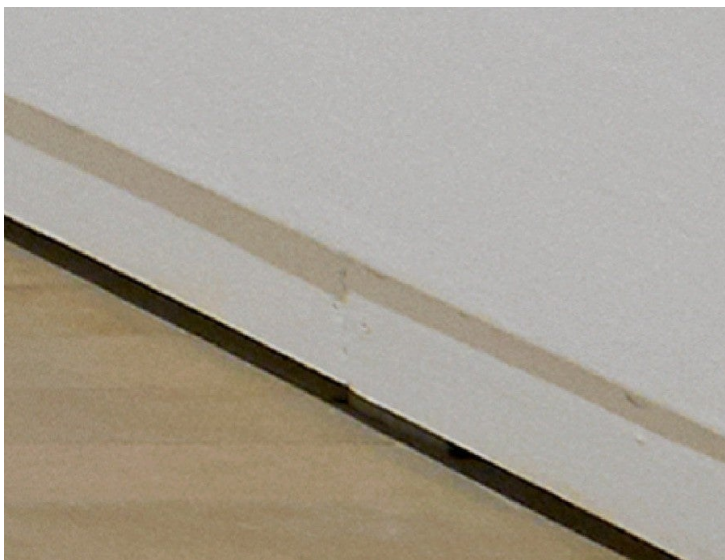
the nails in the skirting of a partition wall;
